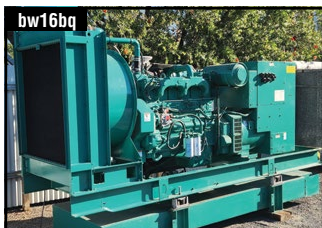
bw16bq GENSET 300KVA CUMMINS, Stam- ford alternator, low hours, serviced and load tested . . . . . $POA
